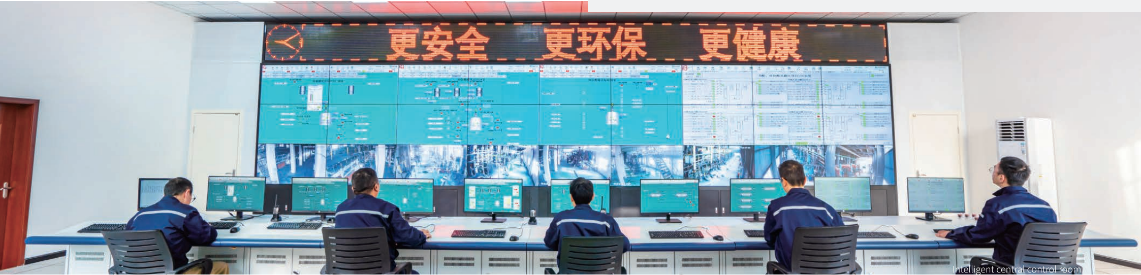
Intelligent central control room
